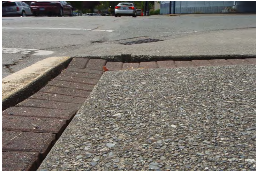
Brick separation along tree wells.
