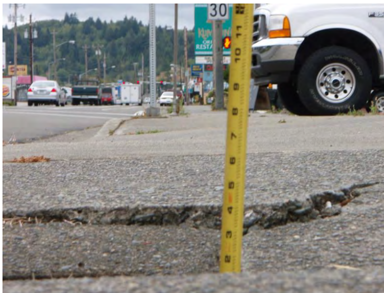
Vertical separation along cracks.
