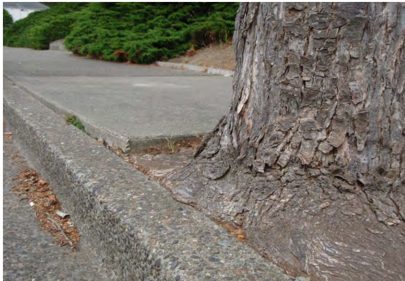
Tree root damage caused to sidewalk.
