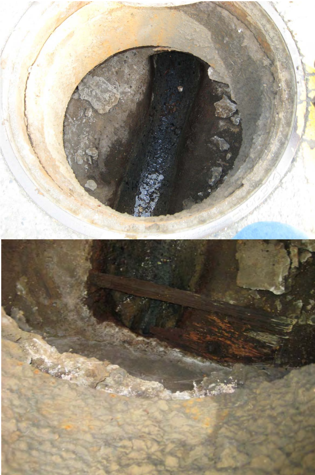
Figure 1.2.4 – Discharge Manhole and Hydrogen Sulfide Evidence
