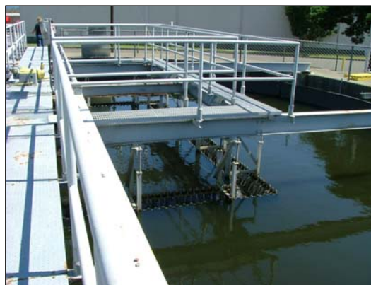
Chlorine Contact Basin
