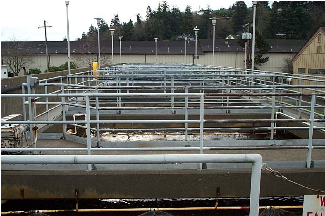
Photo 4 – New primary treatment process installed in 1990.
