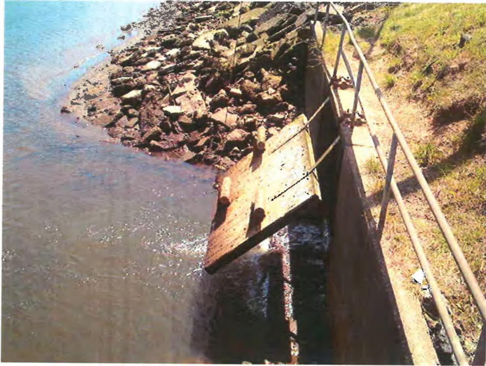
TIDEGATE 12 (Mill Slough Box)
