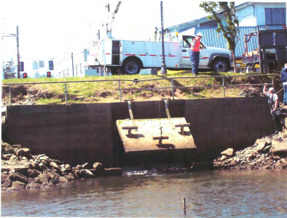
TIDEGATE 12 (Mill Slough Box)
