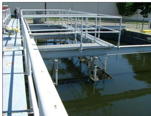
Chlorine Contact Basin
