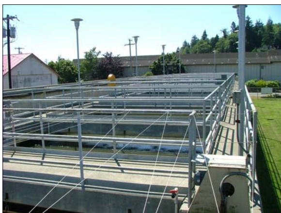
Rectangular Primary Clarifier
